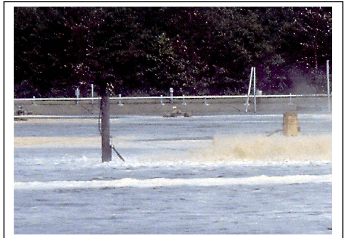
TROLL 8000 installed in a basin
