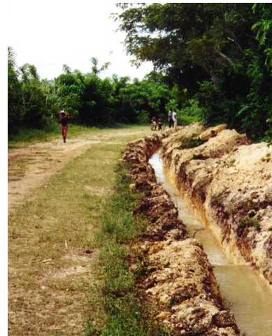
This ditch carries discharge water from the well shown in the photo above to a river located 1 mile to the north. The ditch was necessary so that discharge water would not flood the ag fields.
