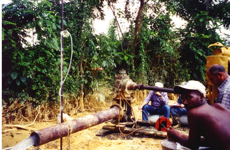
This photo was taken during a pumping test on a new well installed near the freshwater/seawater interface. The test ran for 5 days, during which the pumping rate was gradually increased from 300 gpm to 1200 gpm. Salinity in the well increased at pumping rates above 900 gpm. An MP TROLL 8000 is monitoring water level and salinity in an observation well 14 m southeast of this pumping well.
