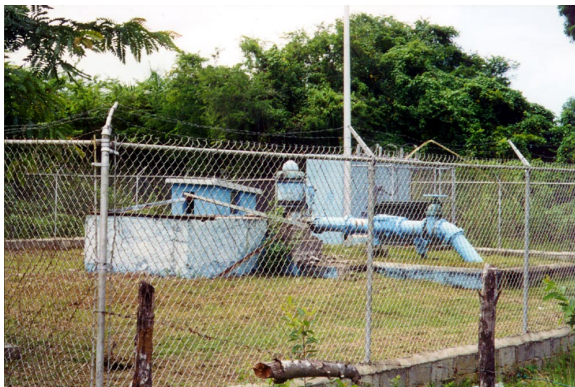
Well #4 in the Los Marenos well field. This is one of the wells being impacted by high salinity, so the pumping rate has been reduced. Capacity = 1800 gpm, Current pumping rate = 1350 gpm, depth = 53 m, screened from 10-53 m - slotted pipe screen.
